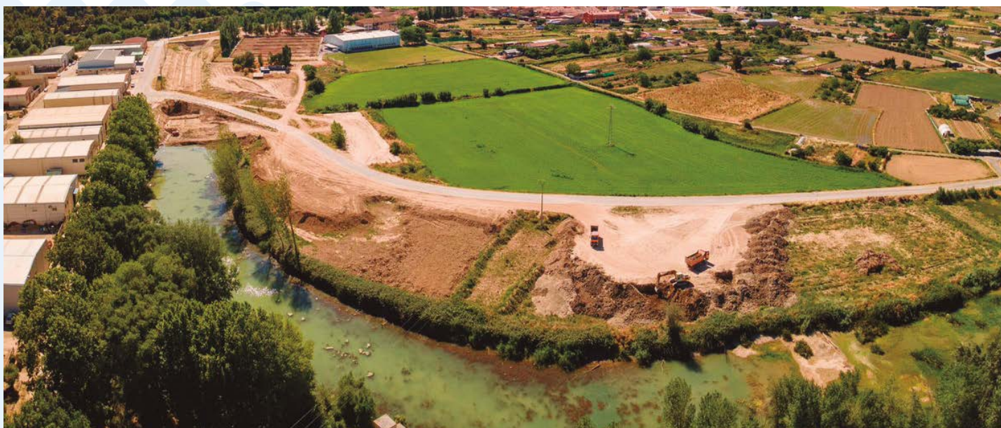
Fluvial restoration of the river Arga in Funes, Ebro basin (Navarra). Connection of abandoned meander of the river Arga
