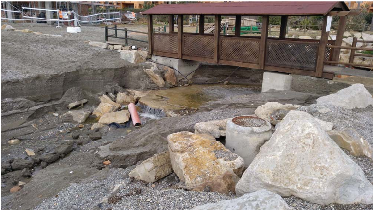
MANILVA: EROSION PLUVIAL
