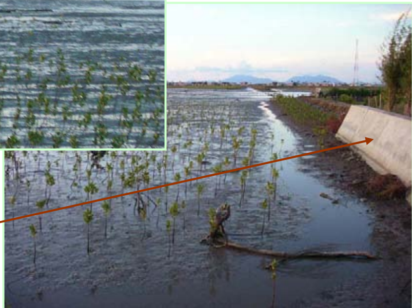
In tact dike walls inhibit natural water flows from land and sea as well as drainage.
